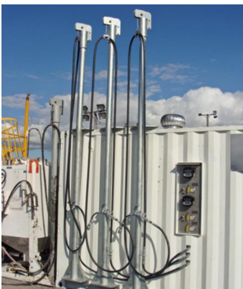
Figure 2 – Remote Dispensing Container with Weighted Hose Towers.
