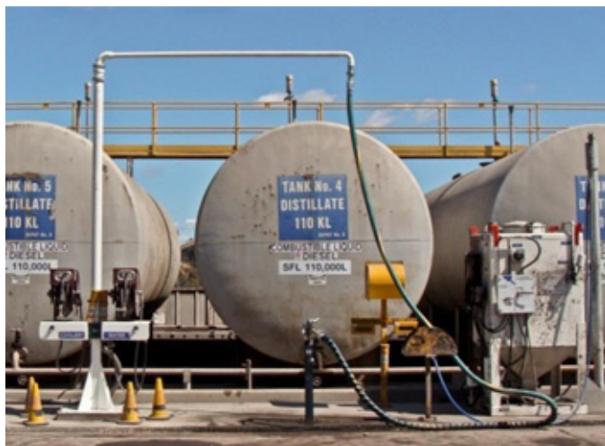
Figure 3 – Diesel Load Out Boom
